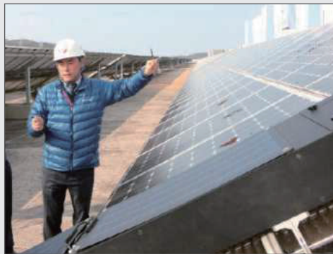
Installation site in power plant
