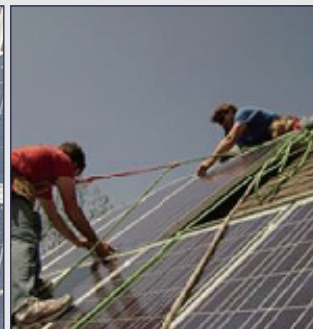
Solar Power Plant built on a high ground
